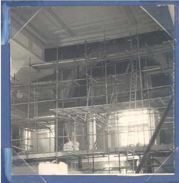
The east end of the church during the construction of the upper chapel and the organ chamber 42
